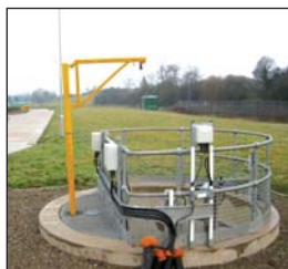
Standard Davit for man-riding and submersible pump lifting
